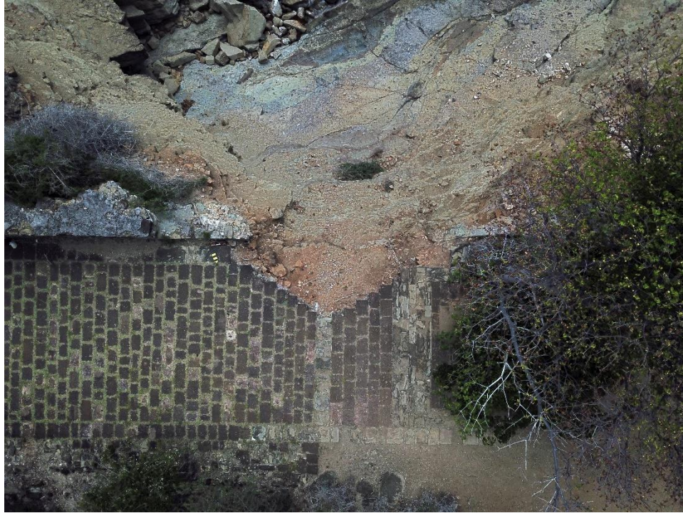
FIGURE 3.2. Aerial view of the eroded wall of Fort Berkeley and underlying cliffside (Photo by DJ Schaefer, ECU, 2022).
