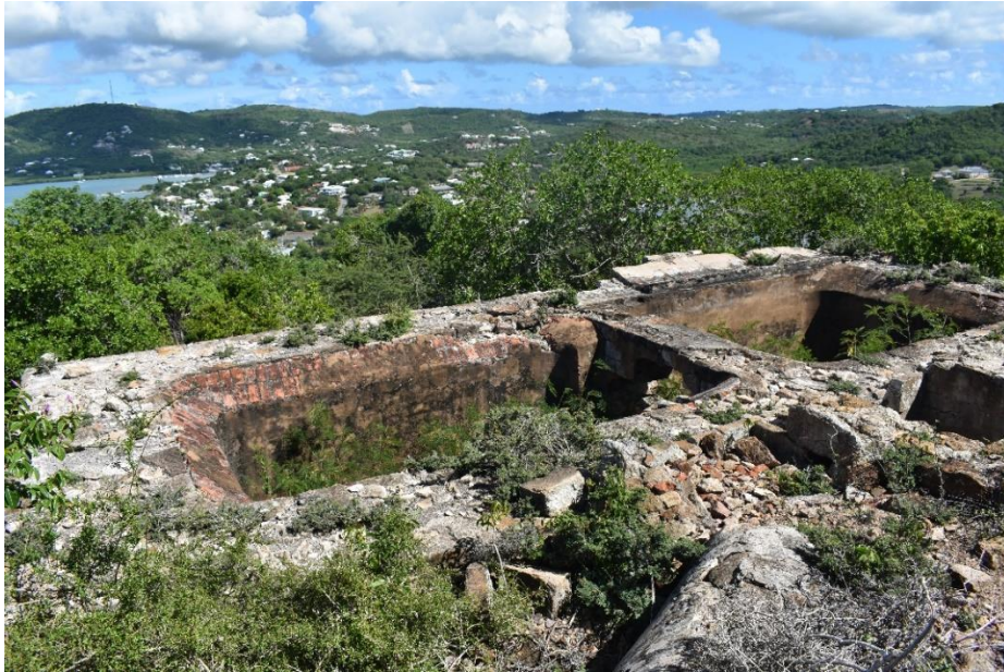
FIGURE 3.4. Perspective view looking northeast of the West India Regiment cistern (Photo by Madison Elsner, ECU, 2022).
