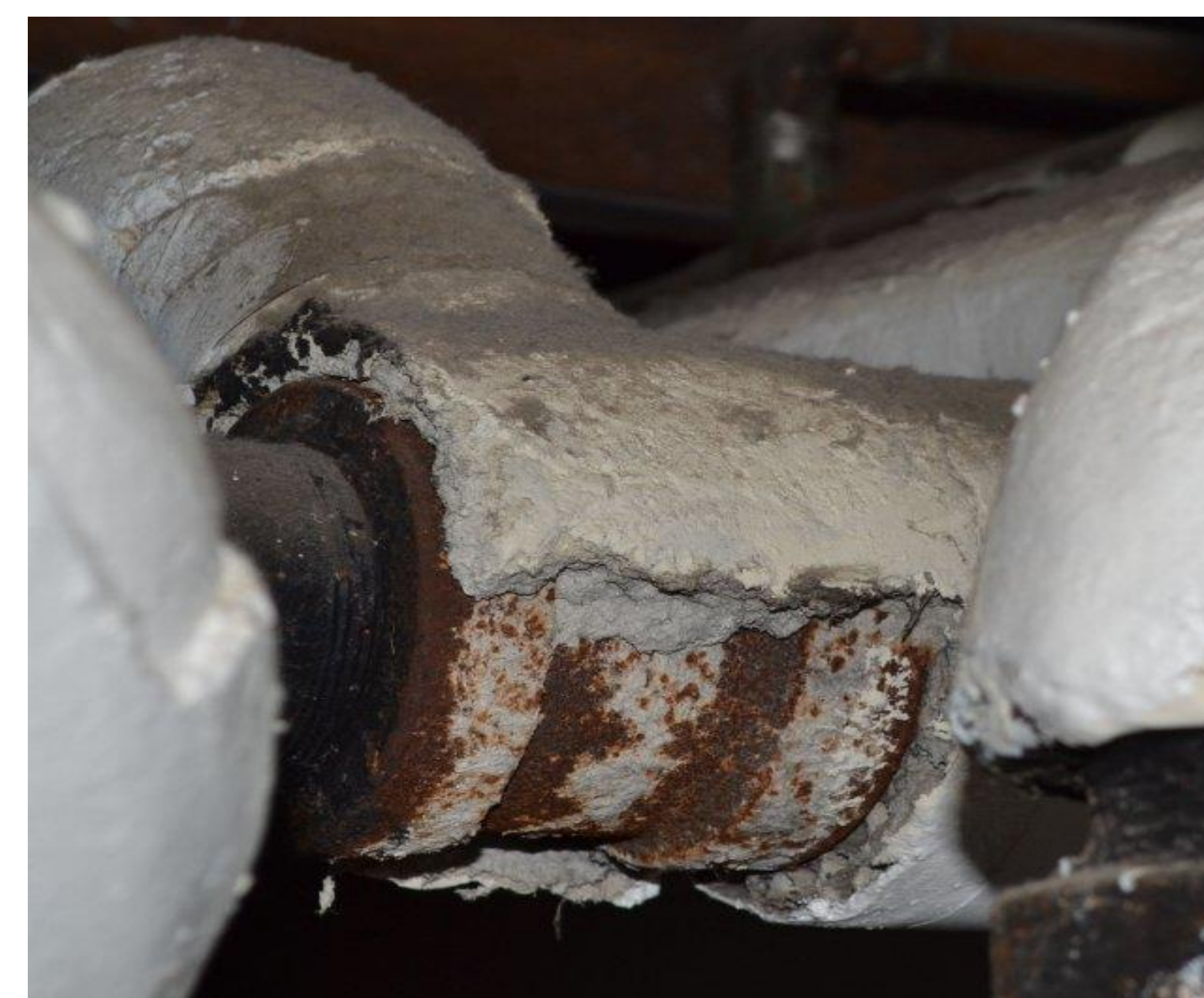
Figure 2. What Asbestos looks like on a pipe installation https://www.epa.gov/asbestos/learn-about-asbestos
