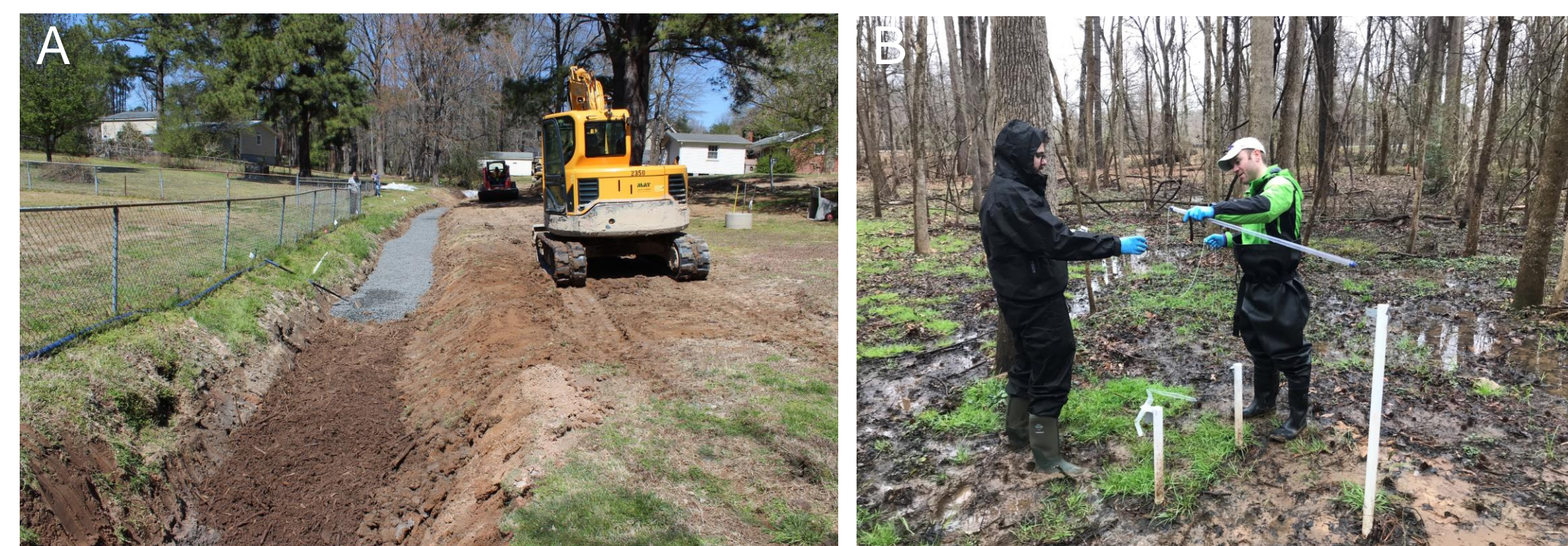
Figure 1. Photos of the in-stream bioreactor during installation (A) and the natural wetland (B).
